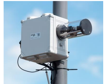
Telescope unit mounted to mast
